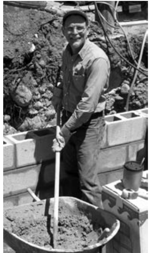
Fr. Dave mixes mortar for the new tool shed, which also serves as storage space and houses water tanks and solar-powered batteries.
